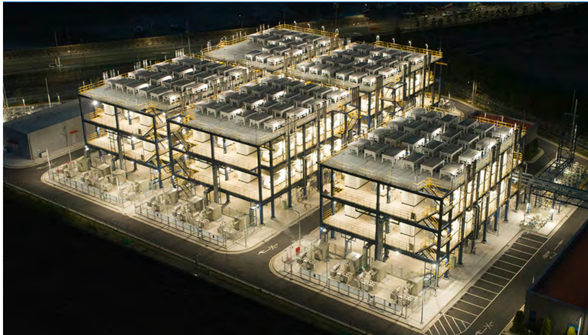
Hydrogen fuel cell power plant
